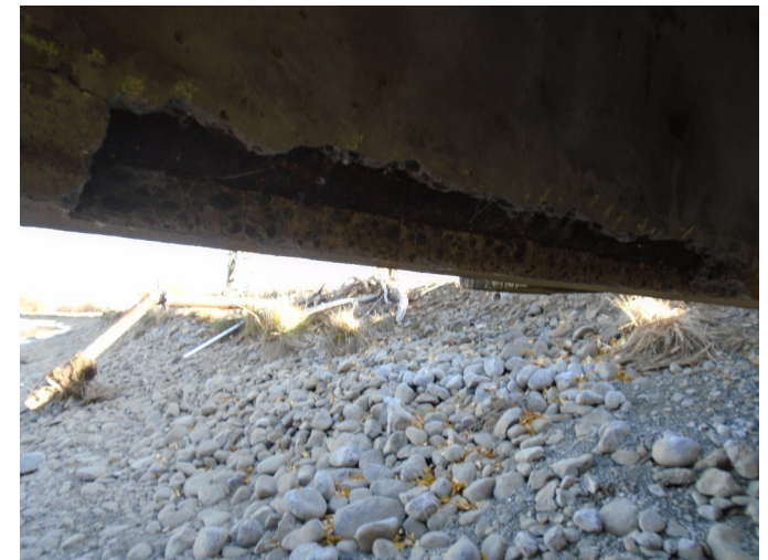
Eroding concrete girder
