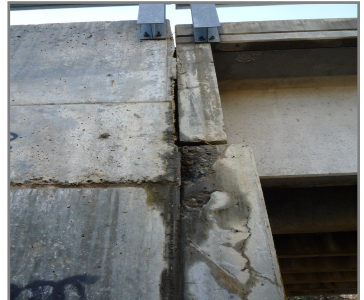
Joint damage visible at inspection
