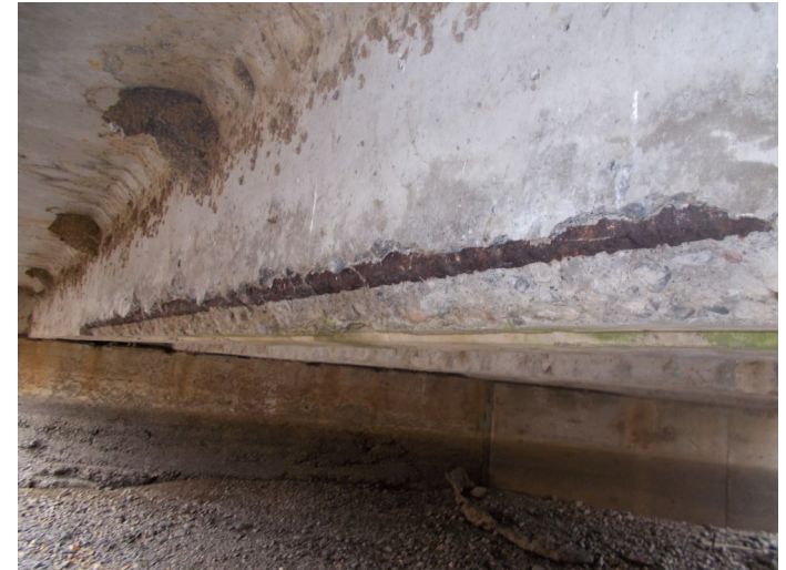
Eroding concrete girder
