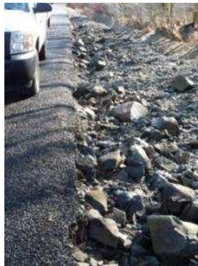
Shoulder Damage from January, 2009 Flooding on Ringer Loop Road
