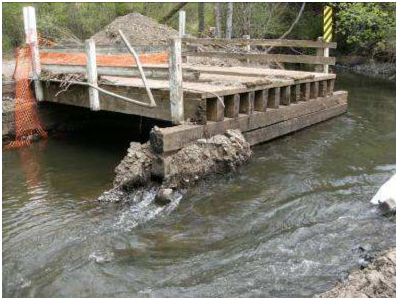
Cooke Canyon Road Bridge after May 15' 2011 Flooding
