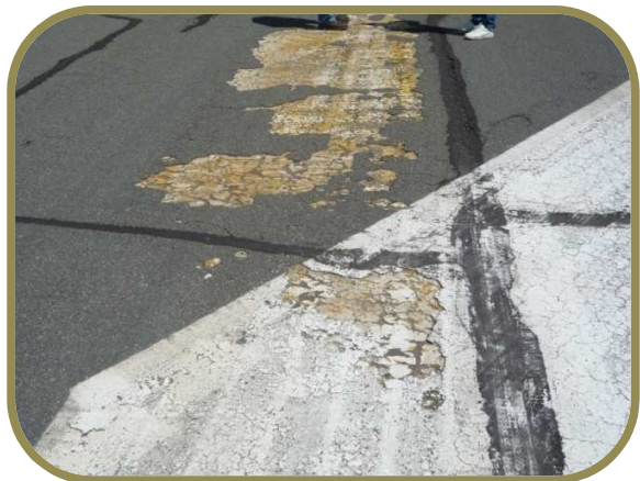
Example of the De-Lamination of the Old Chip Seal
