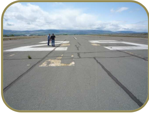
Example of the De-Lamination of the Old Chip Seal
